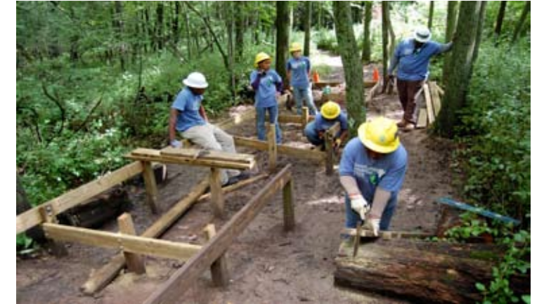
Busy volunteers working on a bridge to span over wetlands on our trails.
